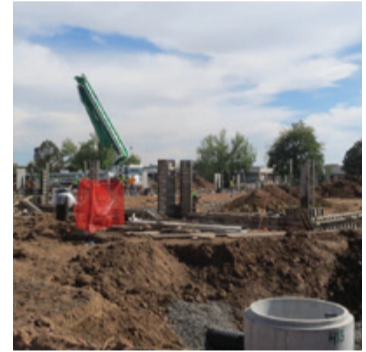
Construction of the Chico's building is underway, with anticipated shell completion by December 2014.
