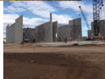
The massive walls for the new state-of-the-art Cinemark Theatre are going up and permits for both the theatre and parking garage have been issued.
