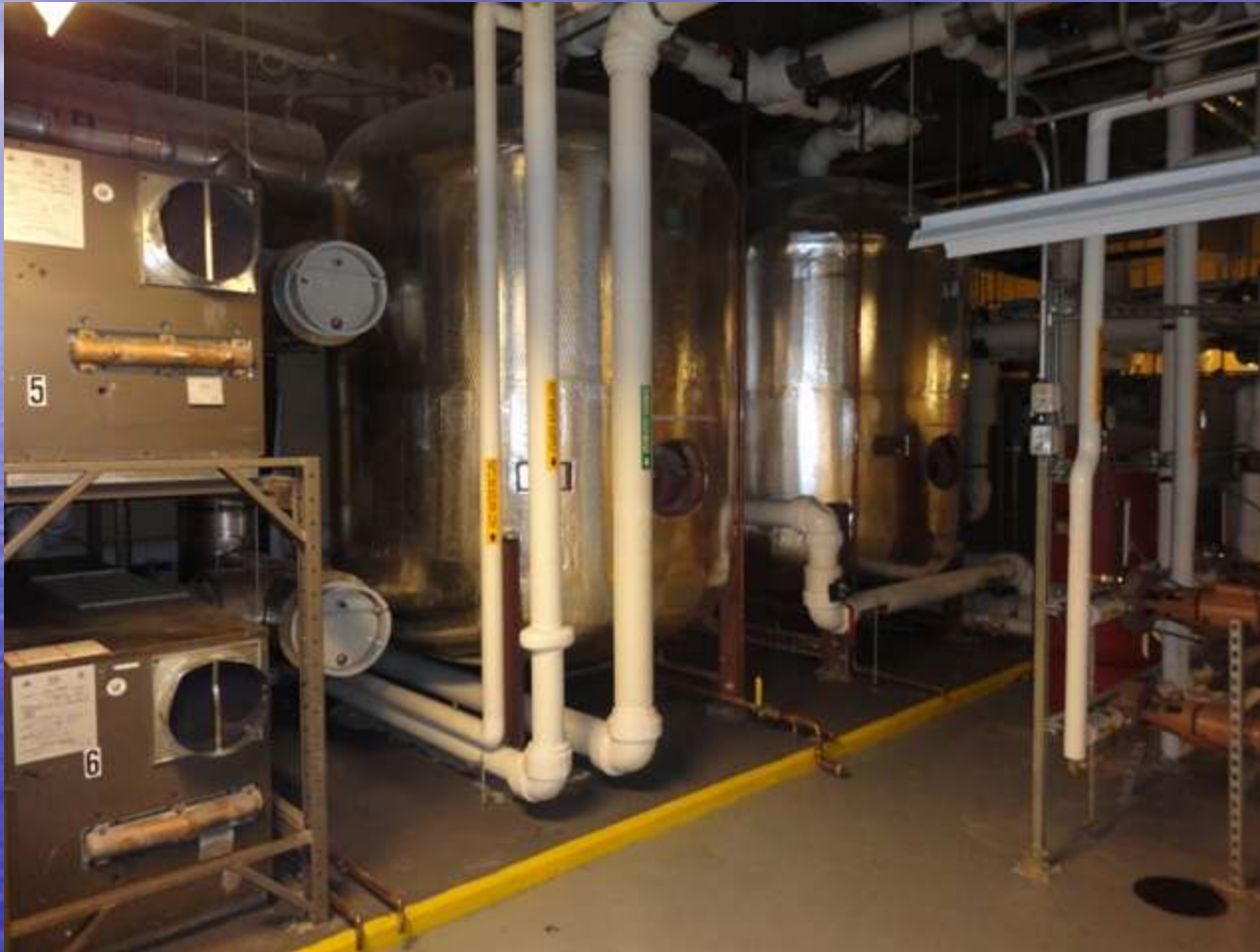
Penthouse hot water storage tanks.
