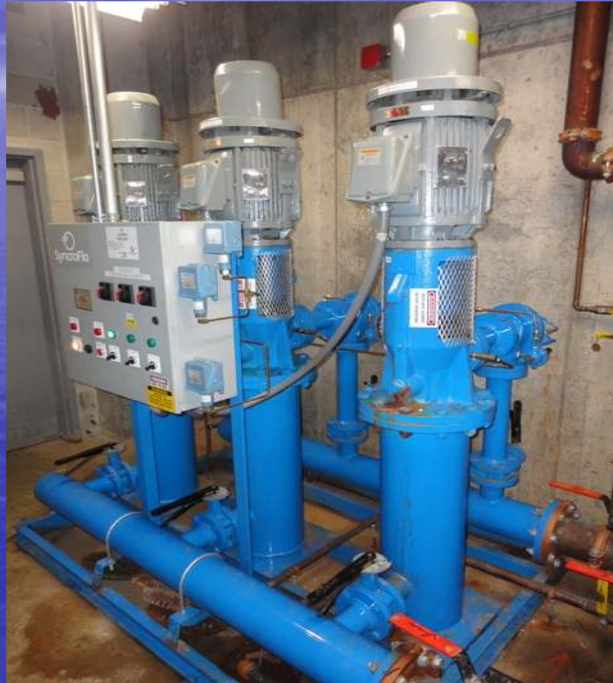
Basement level Water Main Service Room.
