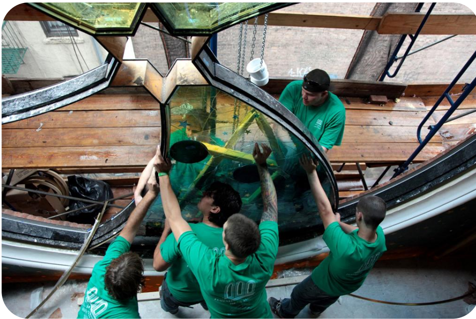
Installation of first panel into the installed frame. Photo courtesy of Kate Milford.
