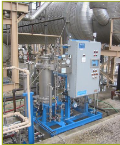
An AmiPur-PLUS installed at Vintage Petroleum, California, USA
