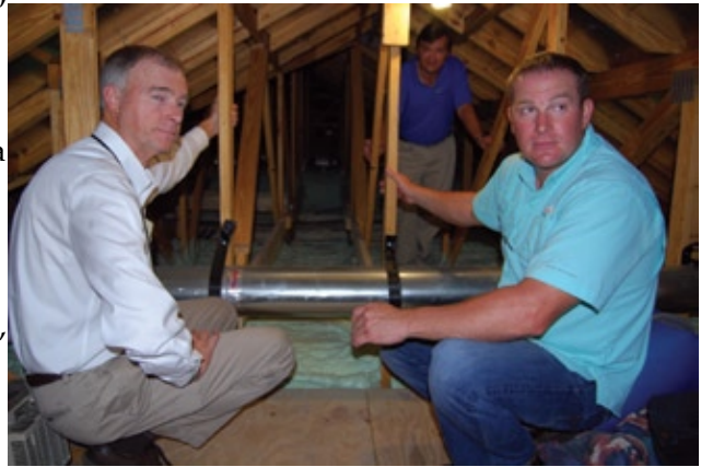
Sherman Phillips and Derek Hembree of Clay Electric are shown with Jason Sheffield, right, in the attic of the Kudlo home. This photo was taken on Sept. 1 in the middle of the day. They spent more than 10 minutes in the attic looking at the insulation and radiant barrier and the temperature was comfortable.
