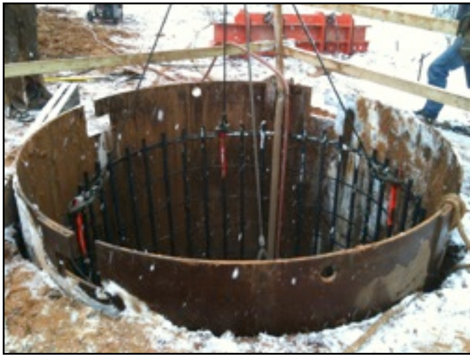
First the foundation of the tower is drilled. A metal casing is used to pour the concrete base.
