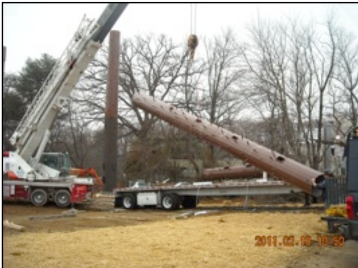
The second part of the pole is lifted with a crane and carefully attached to the “trunk.”
