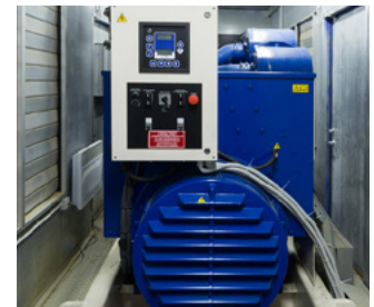
Automatic standby generator
