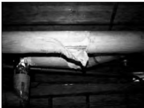
Minor Damage to Pipe Wrap
