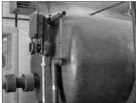
Boiler or vessel insulation
