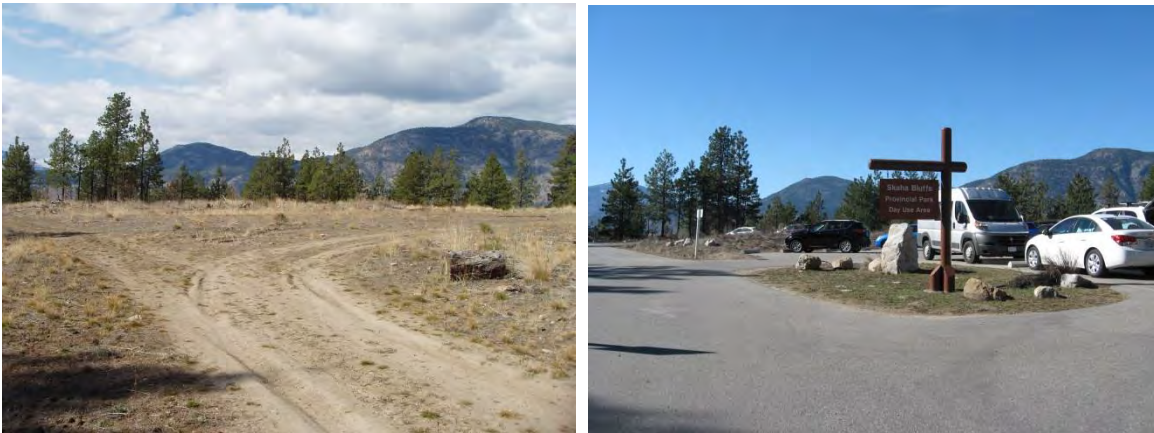
Plate 2: The lower bench parking lot at the time of acquisition in 2008 (left) and fully constructed in 2015 (right).
