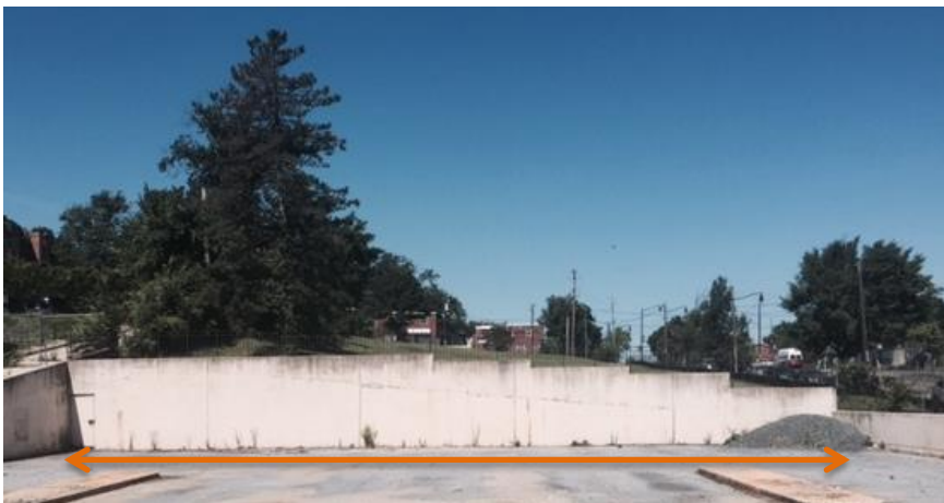
Wall 2 – dimensions: 97' long x 12' tall at highest point The focus of the artwork should be on this wall.
