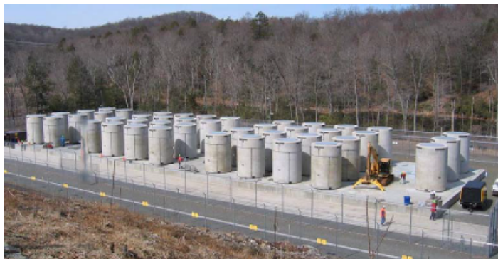
Spent Nuclear Fuel Storage at Connecticut Yankee
