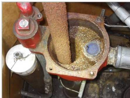
Figure 4: Corrosion found on equipment at one site
