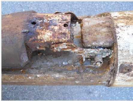
Figure 3: Overfill limiter impaired
