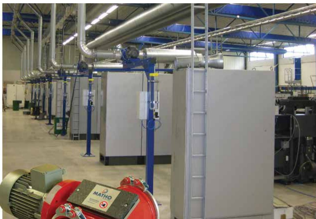
▲ A typical application for a Matho waste management system linking several machines.
